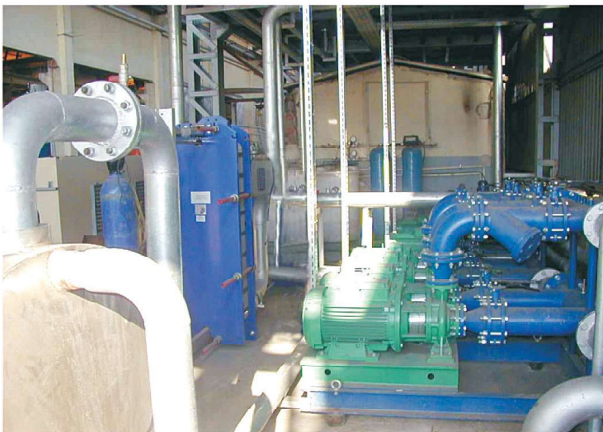
Heat exchanger & Pump station room
