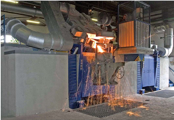
3MW 2x4ton Melt&Hold
