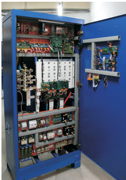
350 kW IGBT power supply (Converter)
